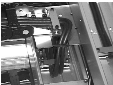
Inside of the junction box
